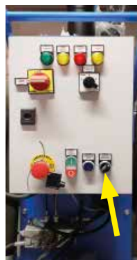
Start/Stop auxiliary pump for particle counter
