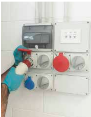
Electrical connection for the three-phase motor (5 poles plug)
