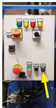
Start/Stop auxiliary pump for particle counter Fig.14
