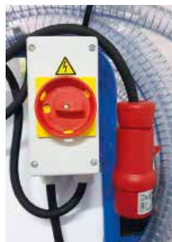
3-phase electrical panel
