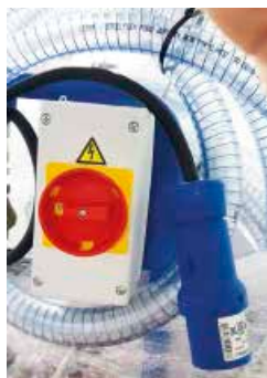
Single-phase electrical panel
